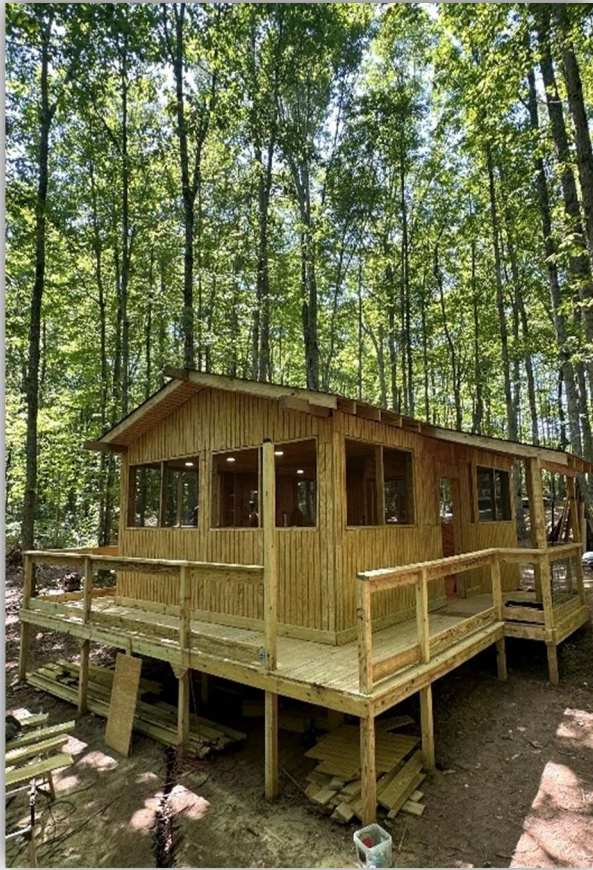
Figure 20. The Appalachian Conservation Institute Bird Banding Laboratory as it nears completion. Photo by Quentin Miller
