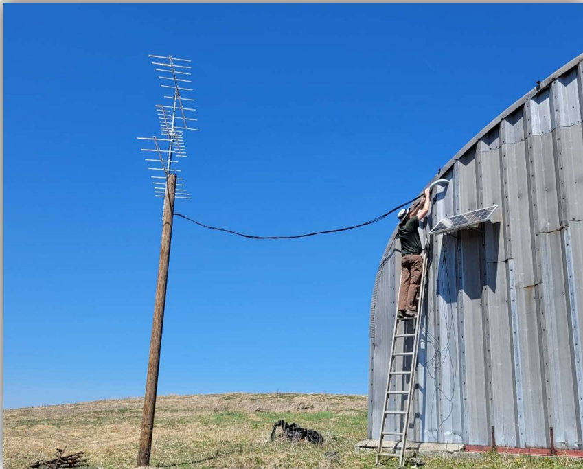
Figure 8. The Pond Mountain Motus Station in Ashe County, NC. Antennas are mounted on a wood utility pole and the station’s battery is charged by a solar panel. The receiver box and battery are housed inside this old airplane hangar. Above, Kendrick Weeks of North Carolina Wildlife Resources Commission runs coaxial cables from the antennas through the side of the hangar building. Photo by Chris Kelly/NCWRC
